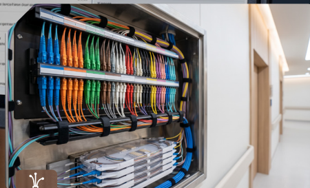
• Fiber Optic Backbone Systems
