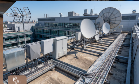
• SMA TV / Satellite TV Distribution Systems
