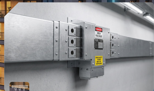
● Busbar Trunking Systems
